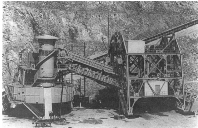
Fig. 13.5.4. Crawlers on movable crusher at a copper installation (courtesy: Dutex, Tucson, AZ).
