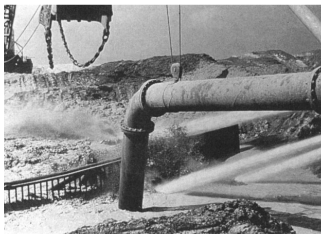
Fig. 14.3.8.3. Well and ore pumping station.
