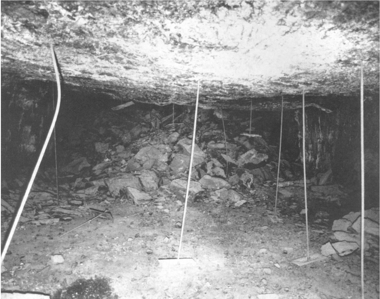
Fig. 10.3.57 View of area of coal mine directly under lineament indicated by arrow in Fig. 10.3.55. This section of the mine has experienced severe bad roof. A growing roof fall extends approximately 100 ft (30 m) back from area seen here (after Peters, 1990).
