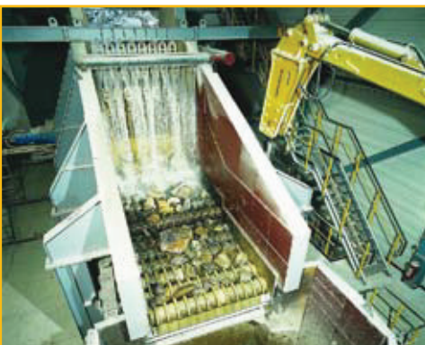
Pre-screening at the Wülfrath-Flandersbach plant.
