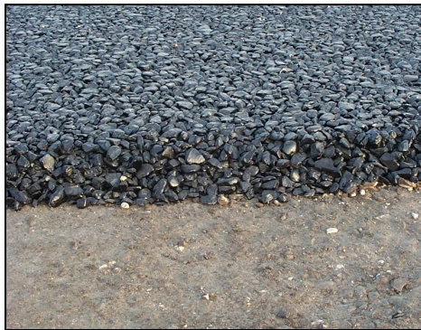
Fig. 3.43. Base layer of asphalt concrete in a road under construction. Gravel is an important constituent.
