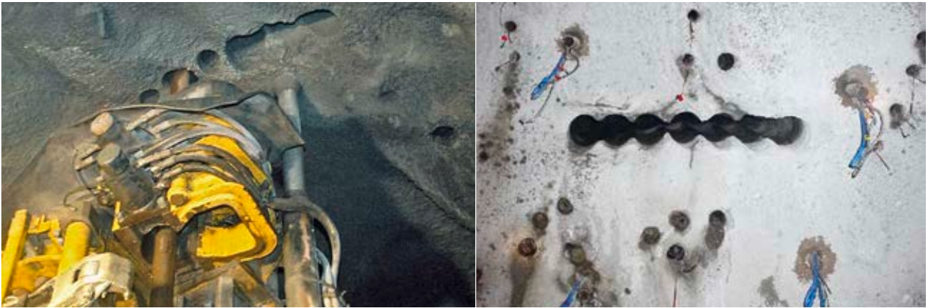
Slot drilling at Ferbasa: The Simba M6 C in action and, (right), the perfectly finished row of holes.
