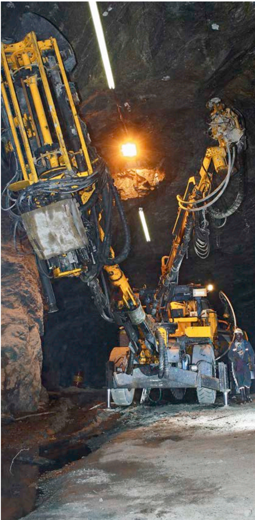
The Cabletec, pictured here at the Otjihase mine, drills, grouts and installs cable bolts.
