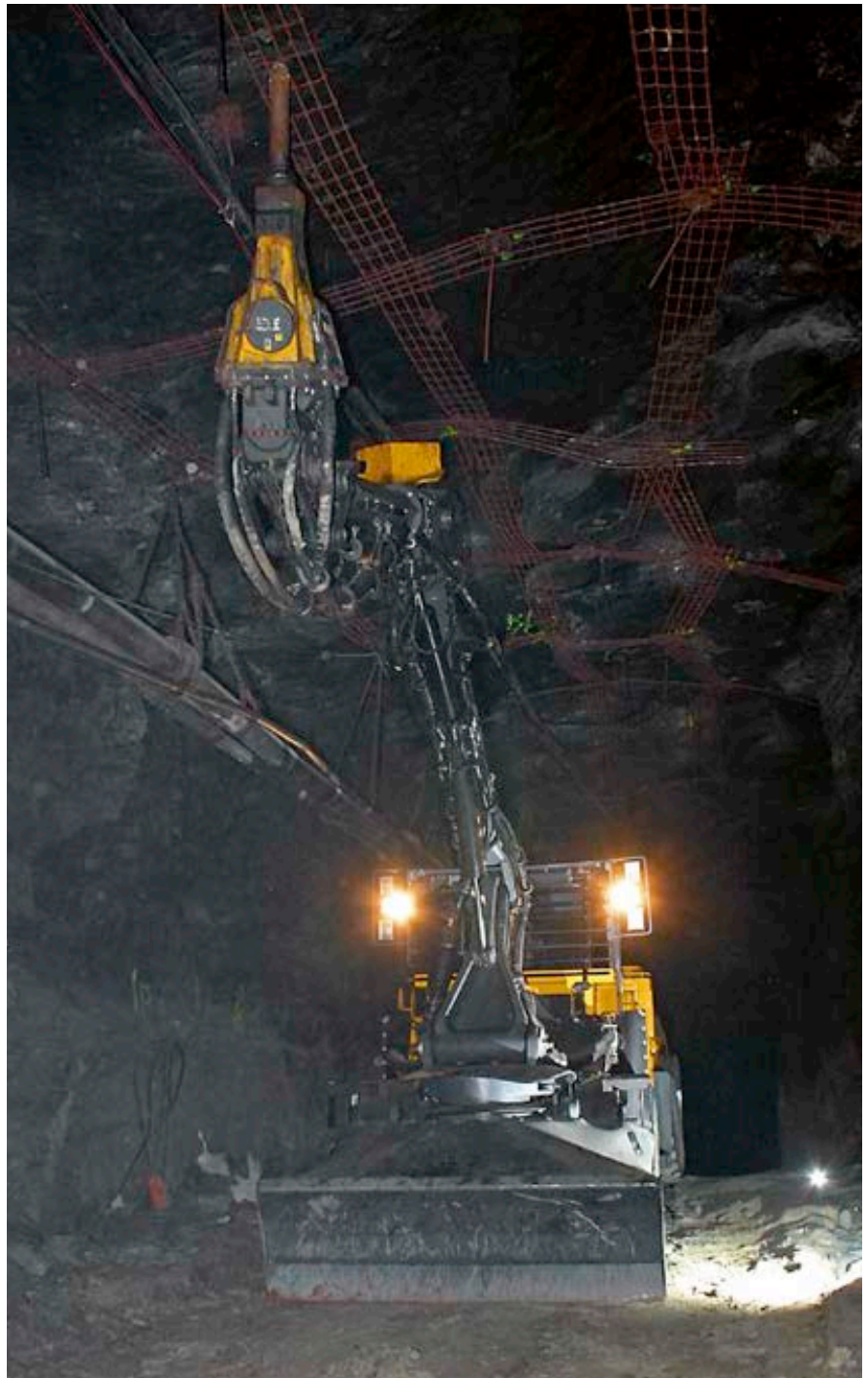
Scaletec MC in operation.
