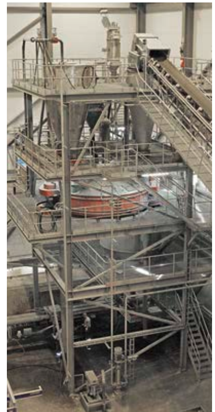
Paste fill plant at Garpenberg, Sweden.
