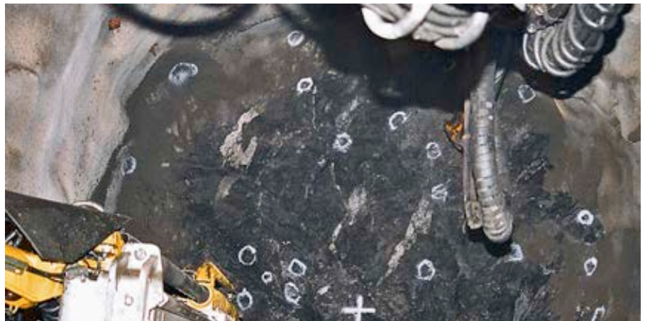
Blasthole markings in stope development at a Tara face, seen from the cab of the Rocket Boomer M2 C drill rig.
