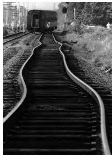
FIGURE 17.7 Thermal expansion distorted these tracks, causing a derailment. Expansion of long structures like this is best described using the coefficient of linear expansion.
