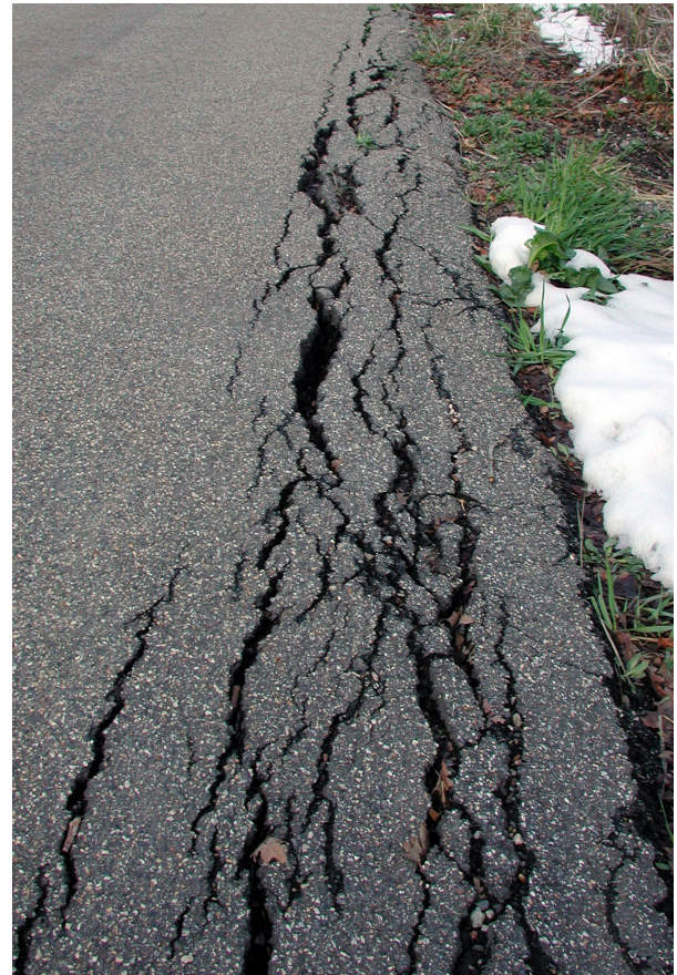
Figure 8.37 Extension fracture population along the edge of a paved road. Each of the fractures have grown from microfractures and have reached a variety of sizes. The pavement is now more or less saturated with fractures, implying that additional strain will accommodate by coalescence of existing fractures rather than by the nucleation of new ones.
